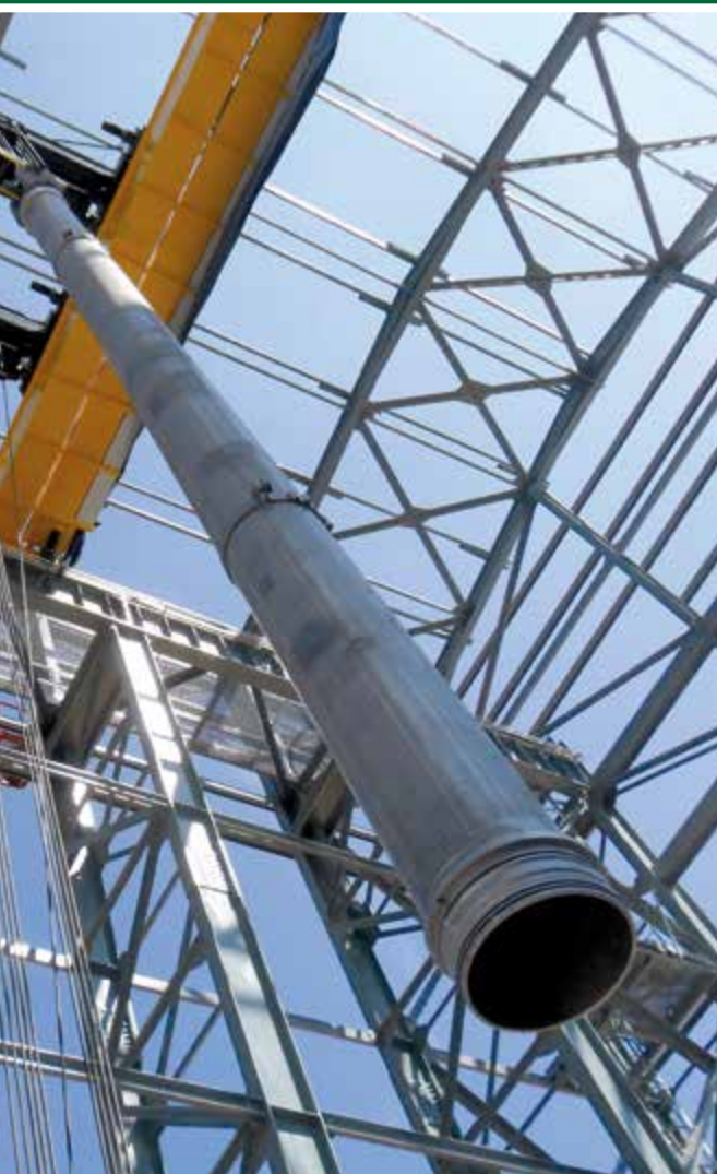
Acid mining dewatering, Johannesburg, South Africa
